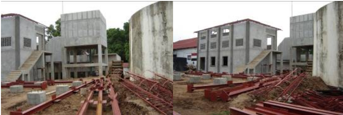
Figure 6: New municipal water treatment plant under construction in Juba city, Southern Sudan
