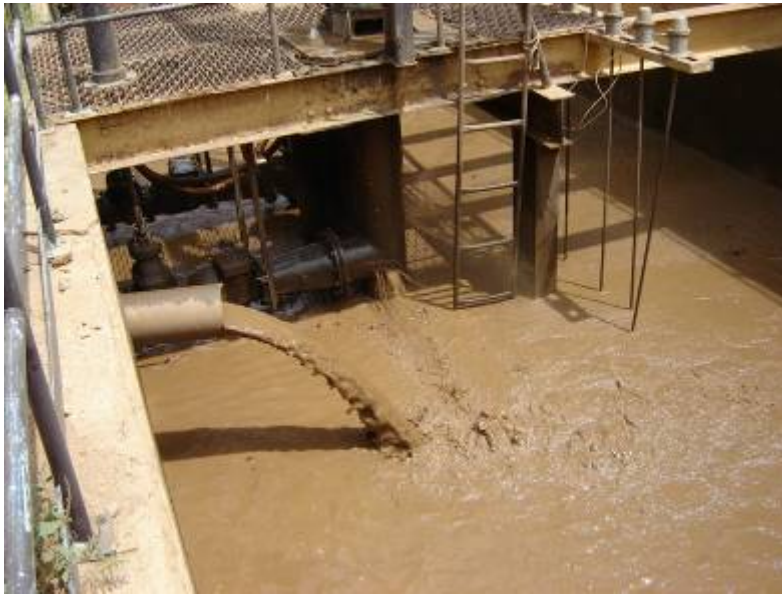
Figure 4: Sludge from flocculator-clarifiers of a treatment plant that is being discharged to the near-by water course.
