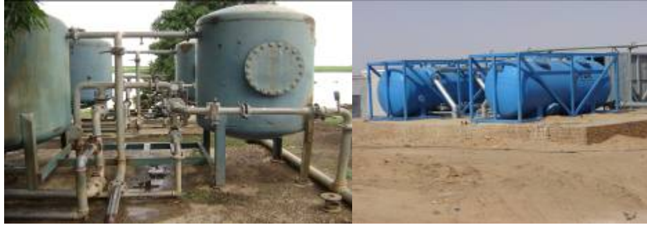
Figure 9: Vertical pressure filter at Malakal, Upper Nile State and horizontal pressure filter at Ousli, Northern State, Sudan
