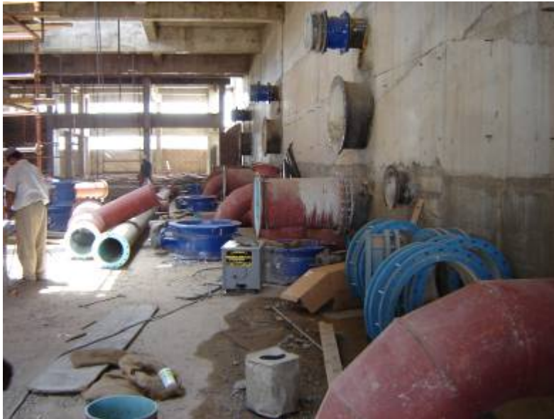
Figure 10: Piping system under construction in a gravity sand filter unit at the New Soba Water Treatment plant in Khartoum
