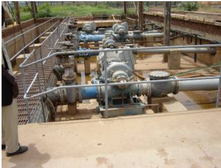
Figure 9: Low lift and high lift pumping units
