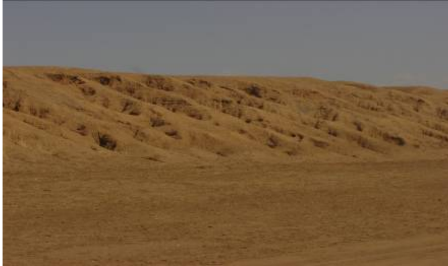
Figure 10: Erosion effect of embankment. Irrigation canal in Kassala State: a good example for the need of regular maintenance of embankment of earth dams
