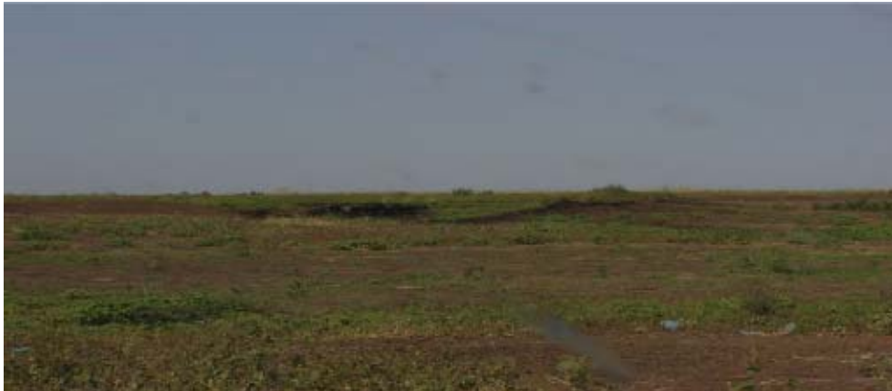
Figure 1. Overtopping of flood water over the body of an earth dam that was caused by a combined effect of high silt accumulation in the storage area and occurrence of high flood. The embankment has been damaged at the left side of the spillway and the dam is not holding the water any more.
