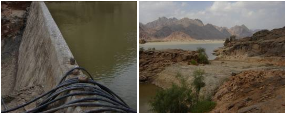
Figure 4. Two spillways for a masonry dam in Red Sea State. (One of them is part of the dam body whilst the other is outside the dam body)
