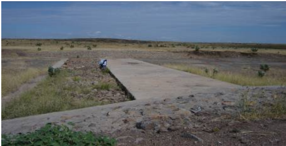
Figure 2. Spillway for the earth dam, constructed outside of the dam body and directed to the nearby natural drainage way
