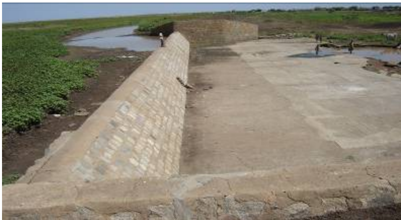
Figure 3. Seepage problem under the free falling spillway of an earth dam
