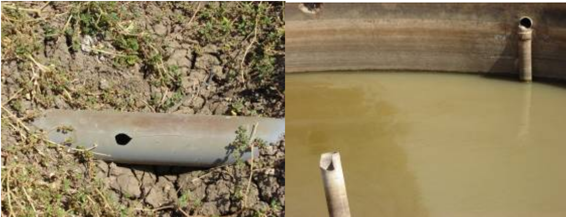
Figure 21. Damaged and leaking supply and connection pipes of sedimentation tank, and filter units at Kerima Al Bahir slow sand filter.
