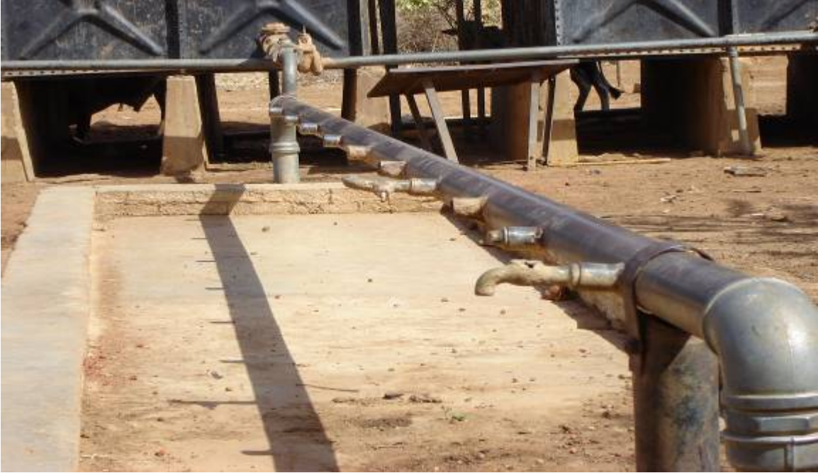
Lack of regular maintenance and replacement of taps makes the system non-functional
