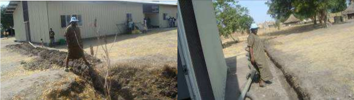
JDF Clinic drainage rehabilitation civil works. Upper picture showing soak away pit.
