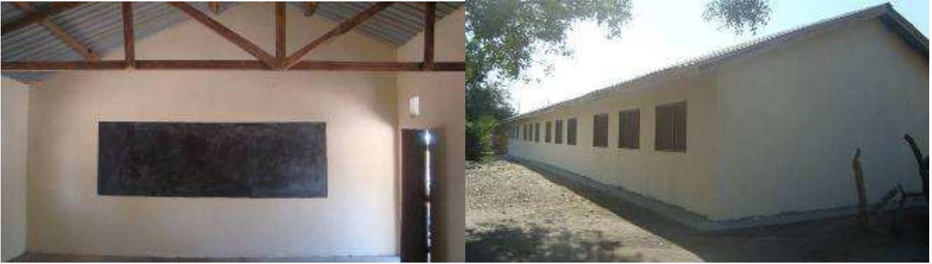
Below are different perspectives including finished classrooms with black board ready for use.
