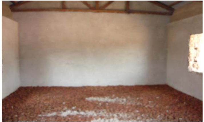
The new interior of a classroom in the block of 4 classrooms and one staff office
